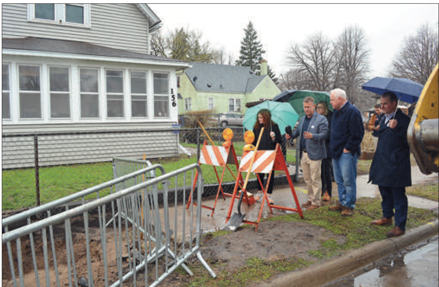
Gov. Tim Walz visited the site of ongoing lead-pipe replacement work in St. Paul, accompanied (L to R) by Rep. Sydney Jordan, St. Paul Regional Water Services Director Patrick Shea and City Council Member Chris Tolbert. Union Advocate photos
