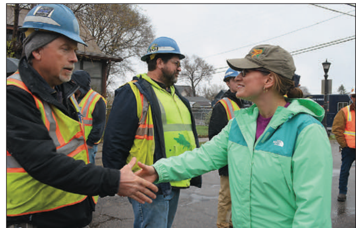
Lt. Gov. Peggy Flanagan greeted a crew of Laborers working to replace lead pipes in St. Paul.
