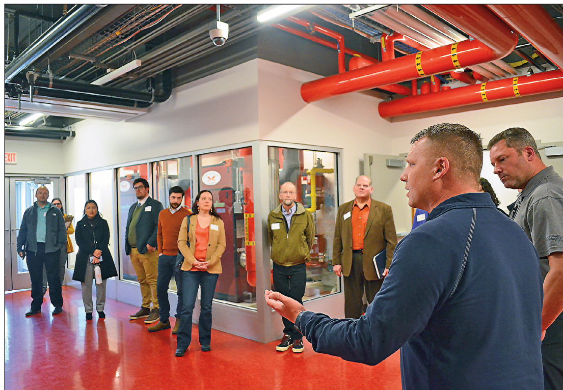
Jeremy McConkey (L), apprenticeship coordinator for St. Paul Steamfitters and Pipefitters Local 455, and Business Manager Tony Poole lead elected officials, civic leaders and city planners on a tour of their training center and its cutting-edge geothermal heating and cooling system. Union Advocate photo
